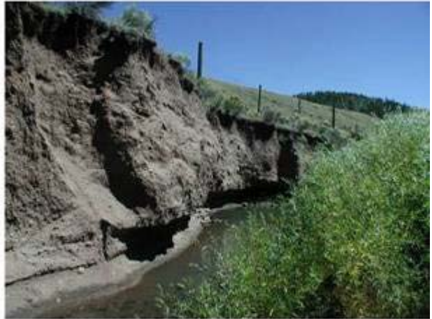
HPP#74 UTM 475232/4070583 Bank erosion point inside enclosure
