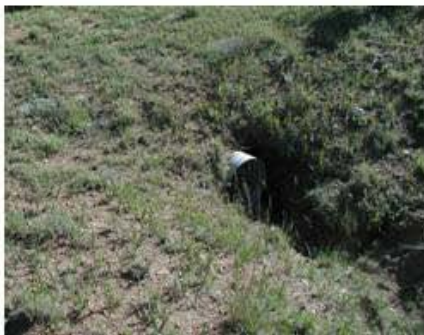
HPR #17-19 UTM 4728773/4073025 culvert/erosion
