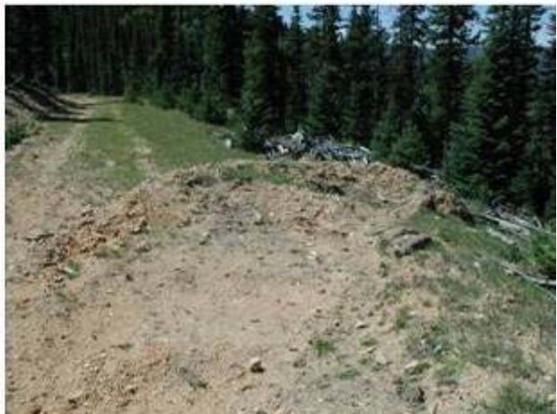
HPP #37 UTM 475453/4076581 water bar adding to erosion
